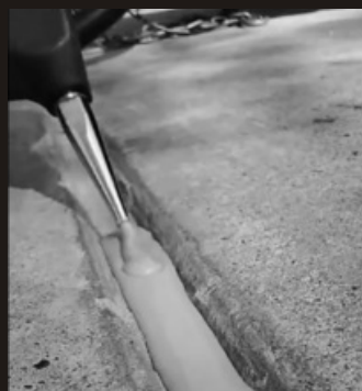
HOT APPLIED MATERIAL
